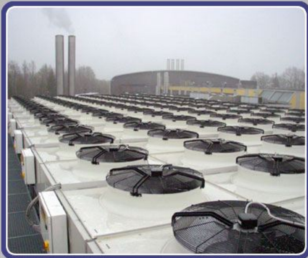
AUSTRIA 10 unit DCS capacity: 4800 kW
