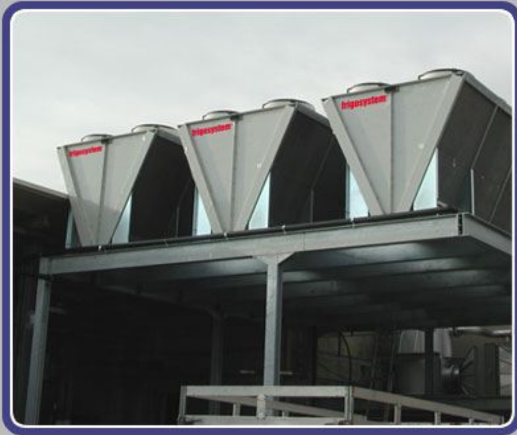
ITALIA 3 unit DCVS capacity: 2800 kW
