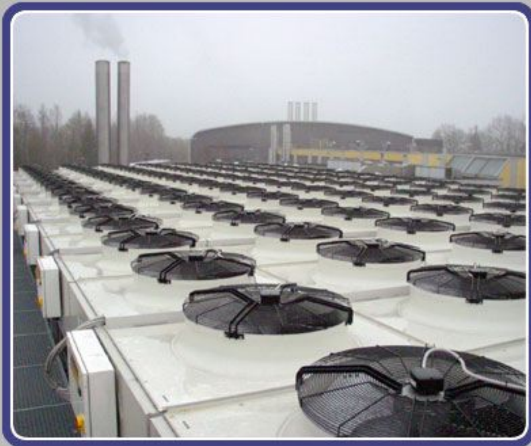
AUSTRIA 10 unit DCS capacity: 4800 kW
